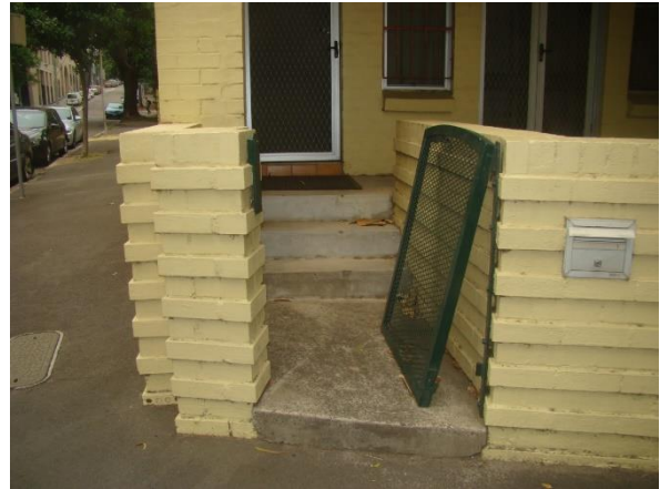
Figure 25. Stairwell at the front of 2A-2D Wentworth Park Road, view looking south.
